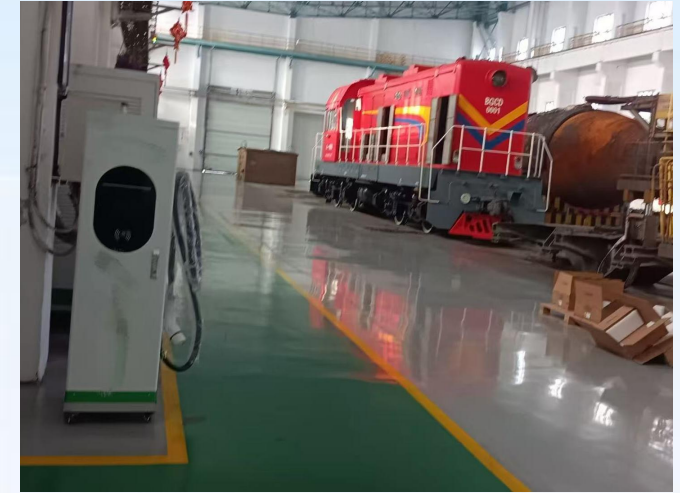
720KW charging stack with two liquid-cooled guns to charge the Xinjiang Bayi new energy locomotive.
