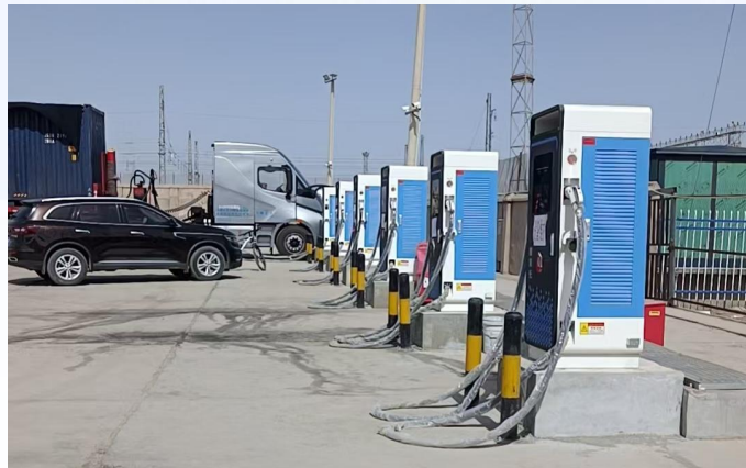
Heavy trucks in mining area of Turpan, Xinjiang, 400KW dual guns charging a truck, high temperature and heavy dust
