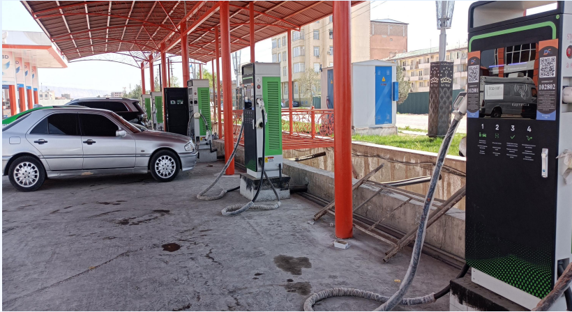
160KW fast charger 6 units in Tajikistan
