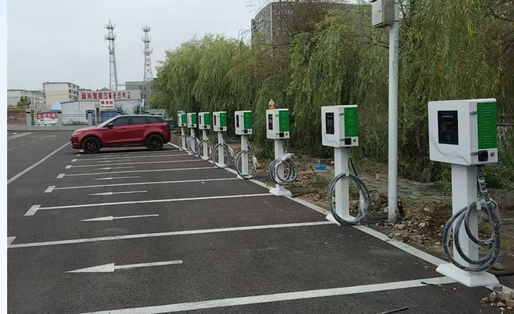
10units 40KW charging stations in Yanji, Jilin
