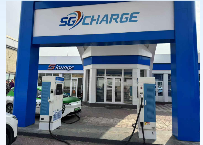
Tajikistan 160KW charging station
