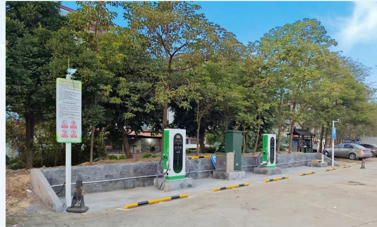
Guangdong government unit 2 units 120KW
